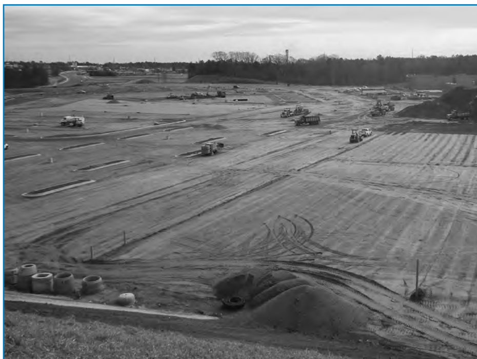
FIGURE 4. WHEN TREES ARE REMOVED AND BURNED TO MAKE ROOM FOR URBAN DEVELOPMENT, THE CARBON IN THE TREES IS RELEASED INTO THE ATMOSPHERE. IN THIS EXAMPLE, THE CARBON BALANCE AND LAND USE ARE AFFECTED. BESIDES TREE REMOVAL, IDENTIFY ONE MORE SOURCE OF ATMOSPHERIC CARBON DIOXIDE IN THIS PHOTO.
